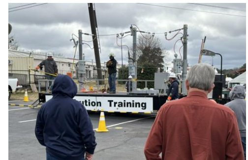
Duke Energy Live Line Demonstration
